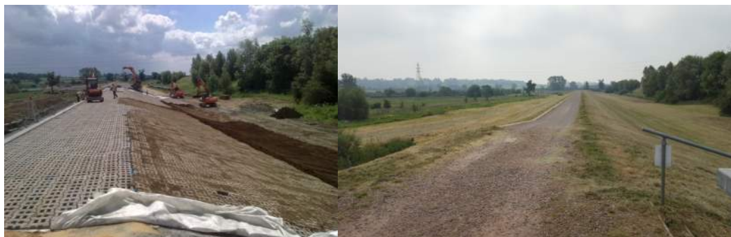
Figure 7-1: Grass Covered Articulated Concrete Block Slope Reinforcement, During Construction (left), Post Construction (right)
