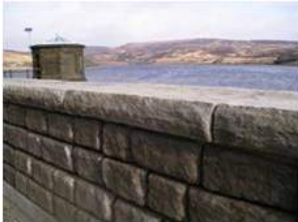
Figure 7-3: Redi-Rock wave wall at Walshaw Dean Reservoir (photo reproduced with permission of CPM Group)
